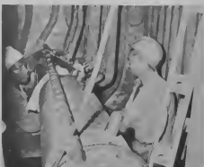
WORKING IN confined space, these men install 144 tubes for the superheater. TRAHANDO DEN espacio perta, e trahadornan aki ta instala 144 tubo pa e superheater.
